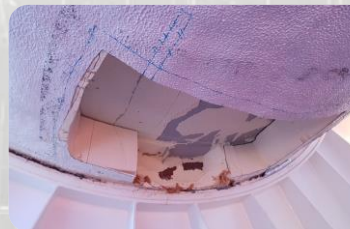
Crack & Delamination due to Shrinkage & Movement
