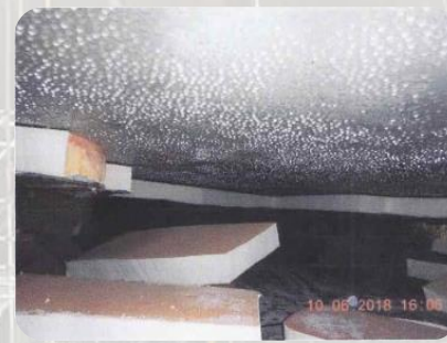
Delamination & Fall Off
